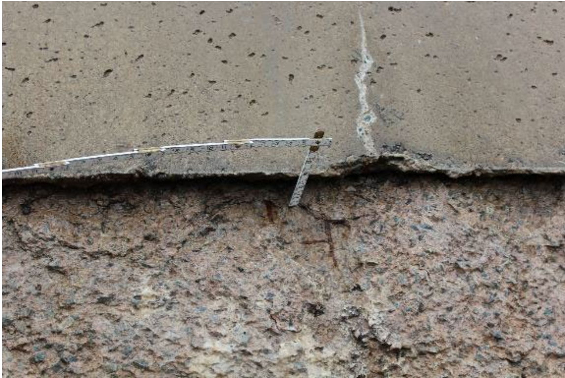
Photo 23: Depth of erosion at top of third facing element above bottom of spillway
