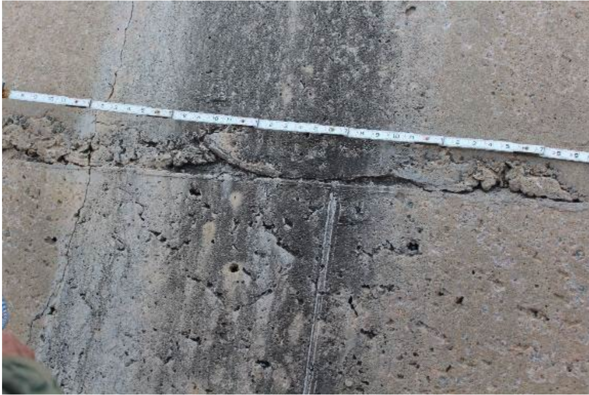
Photo 14: Poor consolidation at horizontal joint between facing panels
