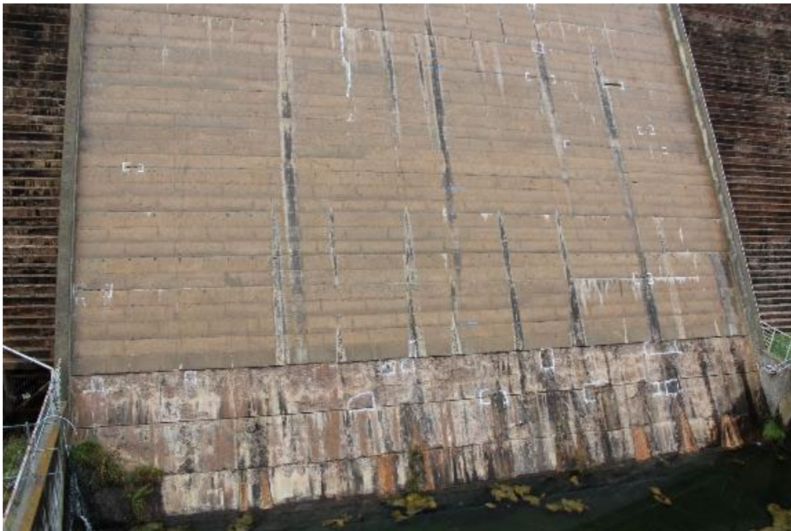
Photo 21: Deteriorated and delaminated areas on spillway lower facing elements
