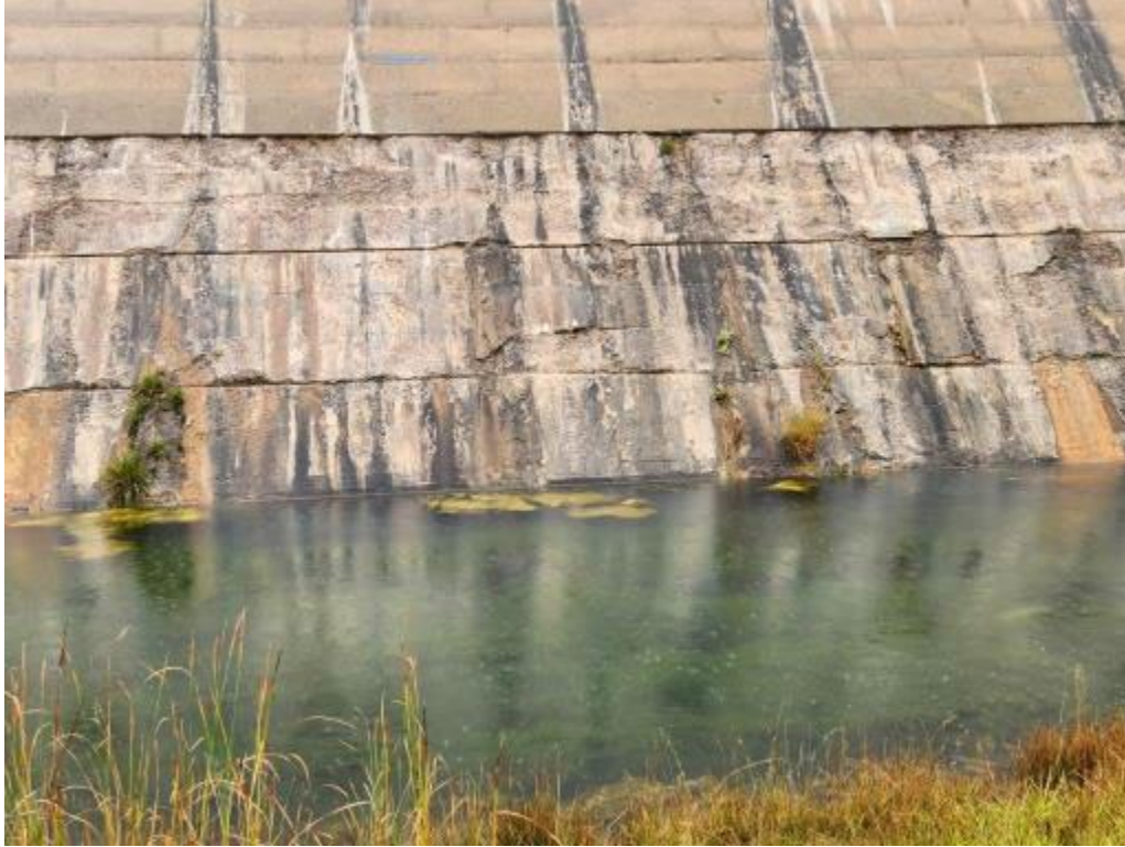
Photo 20: Deteriorated facing panels on bottom of spillway
