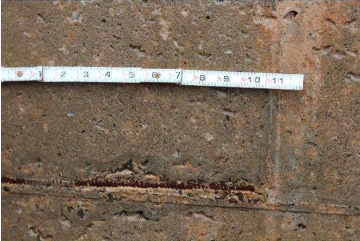
Photo 10: Rebar exposed on spillway concrete surface (Field Note 22)
