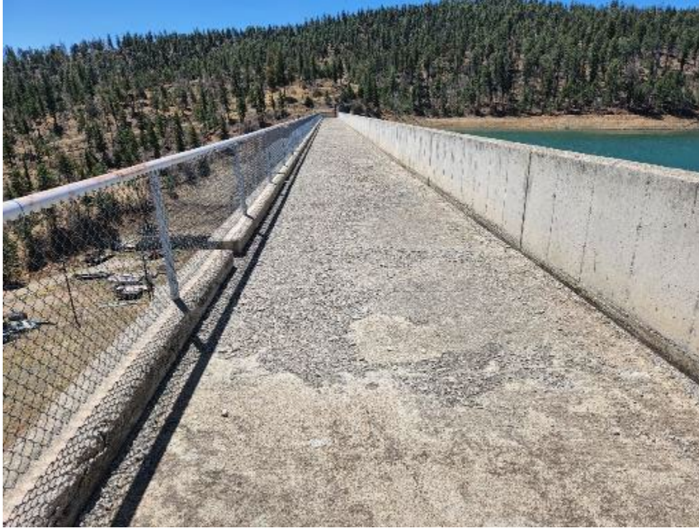
Photo 36: Transition from deteriorated concrete to good concrete on the dam crest.
