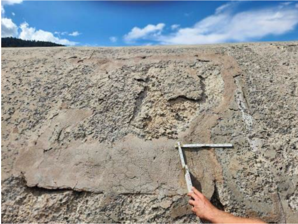
Photo 5: Dam crest drummy concrete surface delamination
