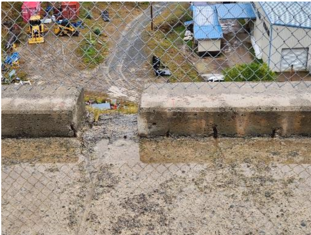
Photo 31: Exposed rebar along side of curb on dam crest
