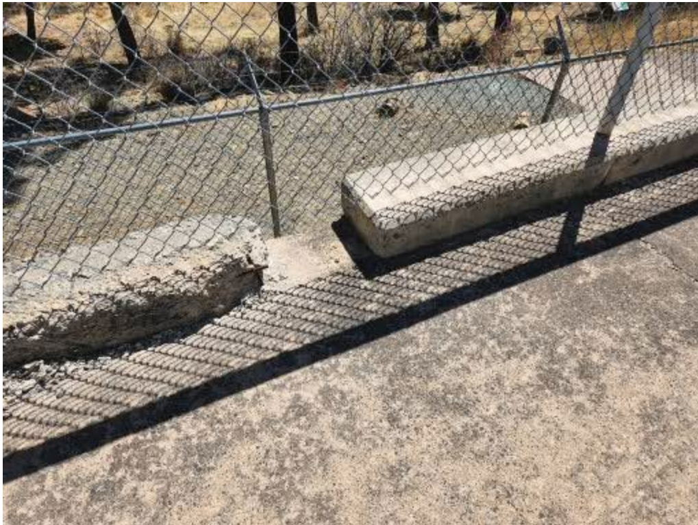
Photo 33: Change from severely deteriorated curb to non-deteriorated curb on dam crest
