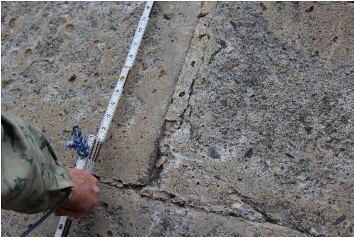
Photo 11: Deterioration and spalling at vertical joint on spillway surface.
