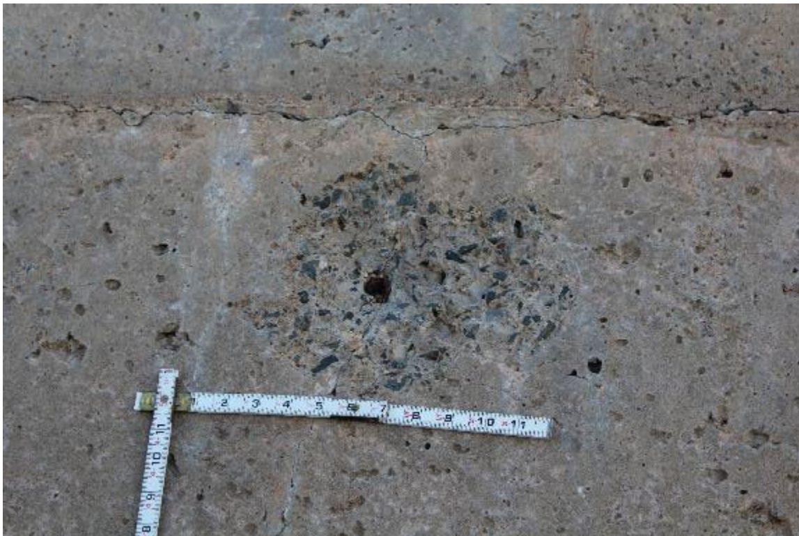
Photo 19: Spalling at embedded form insert on spillway
