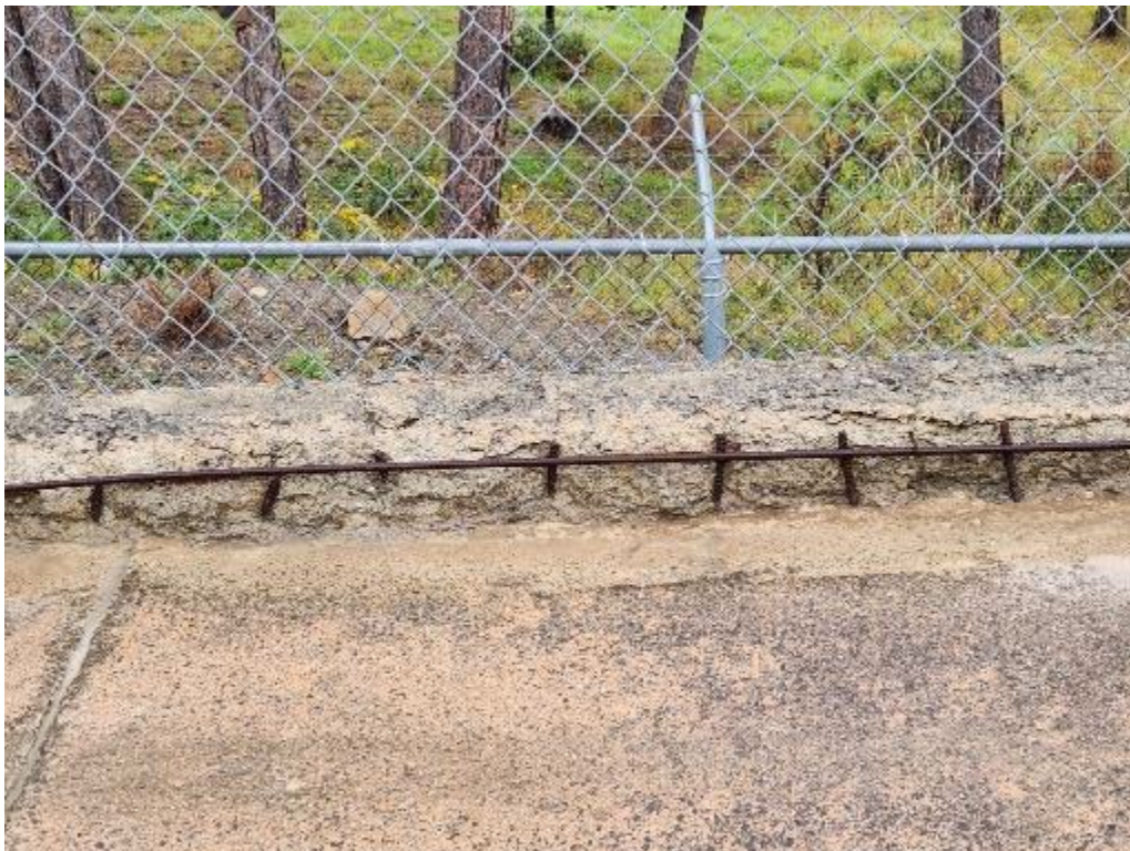
Photo 25: Deteriorated curb and exposed rebar on dam crest
