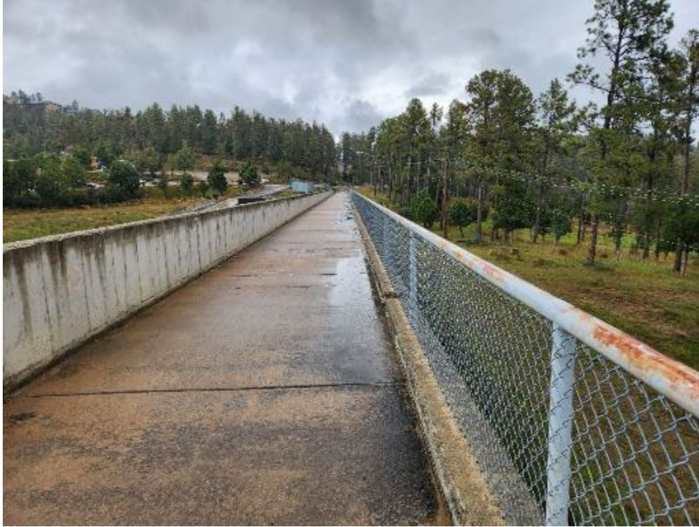
Photo 32: Ponding at curbs on dam crest
