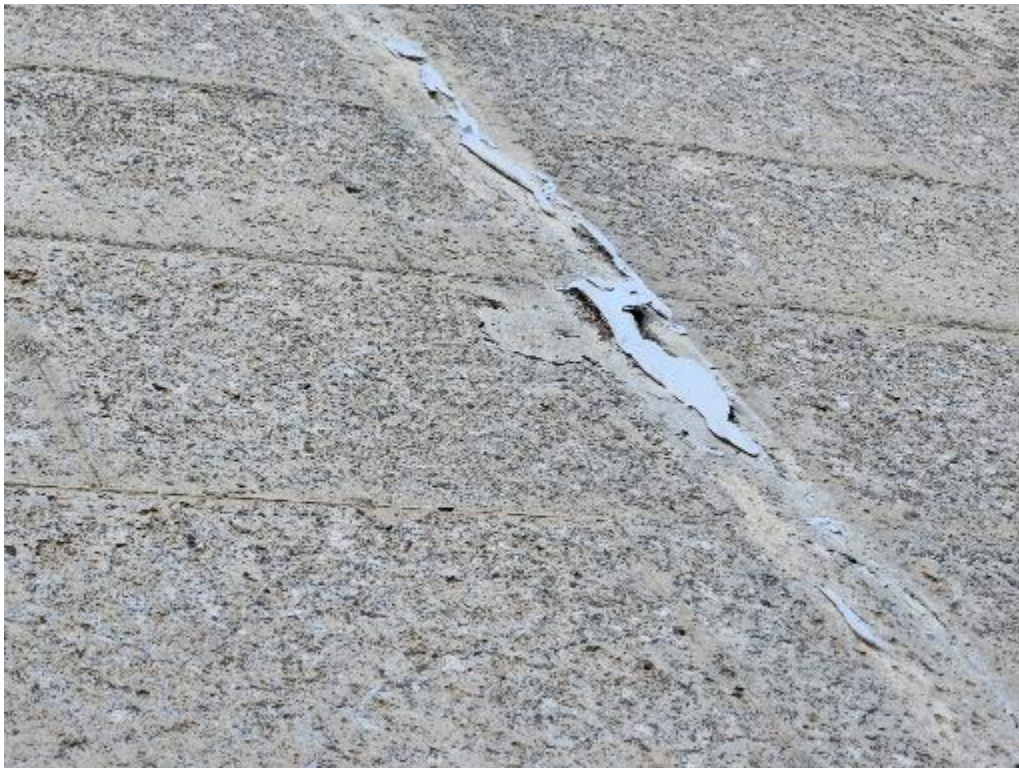
Photo 7: Failed crack repair (Field Note 5)
