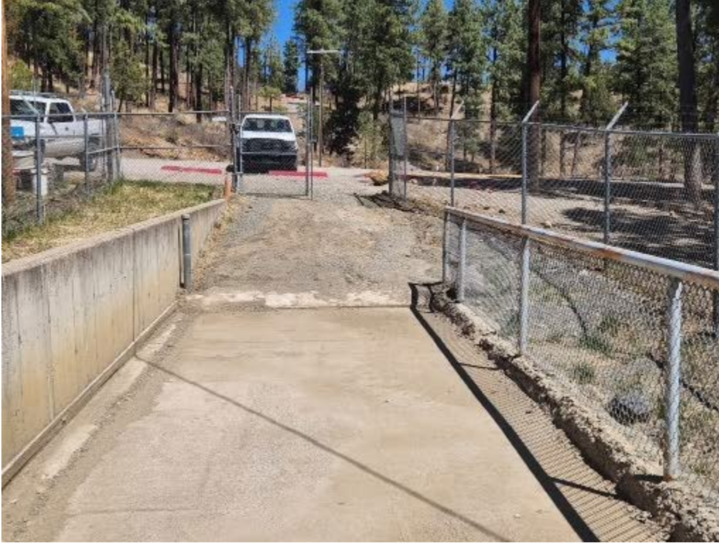
Photo 26: Severely deteriorated curbs at north end of north dam crest
