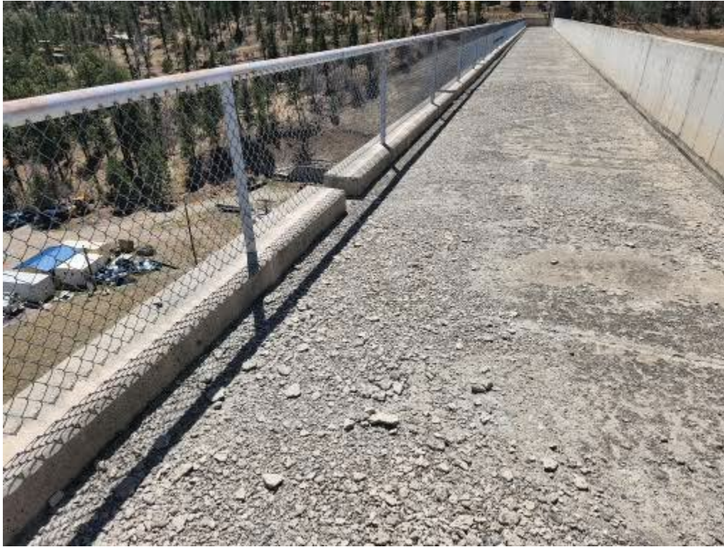
Photo 34: Deteriorated concrete surface on dam crest
