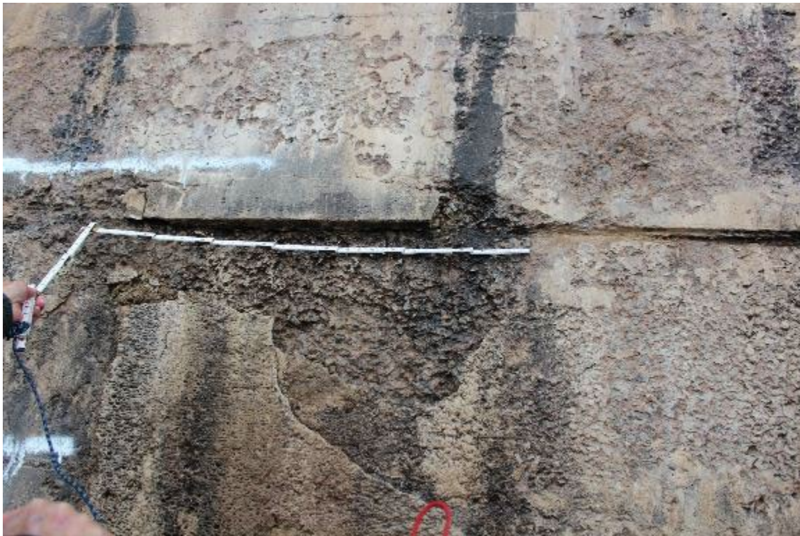
Photo 17: Erosion on concrete surface on lower facing elements
