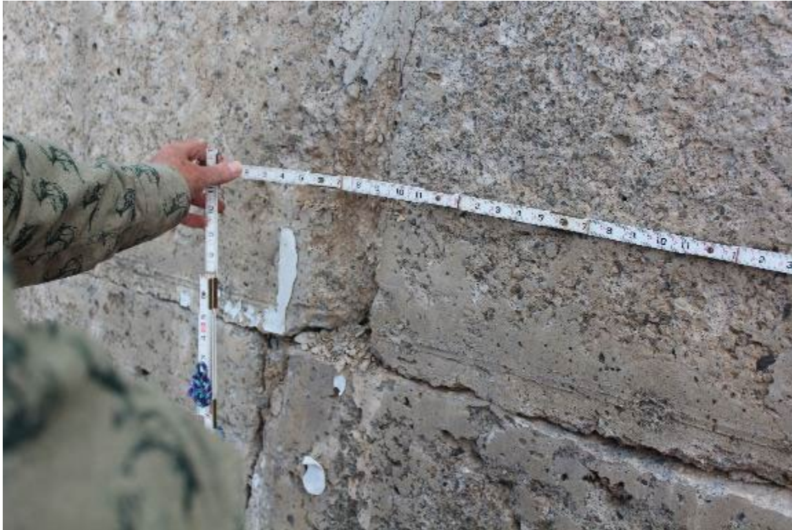
Photo 8: Spalling at vertical crack on spillway
