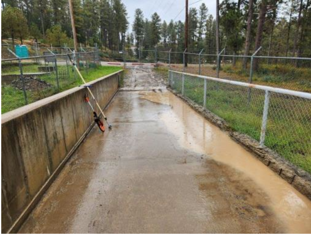
Photo 28: Severely deteriorated curbs and ponding on north end of north dam crest
