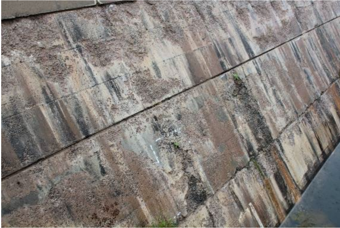
Photo 22: Deteriorated facing elements at bottom of spillway (note horizontal form lines)
