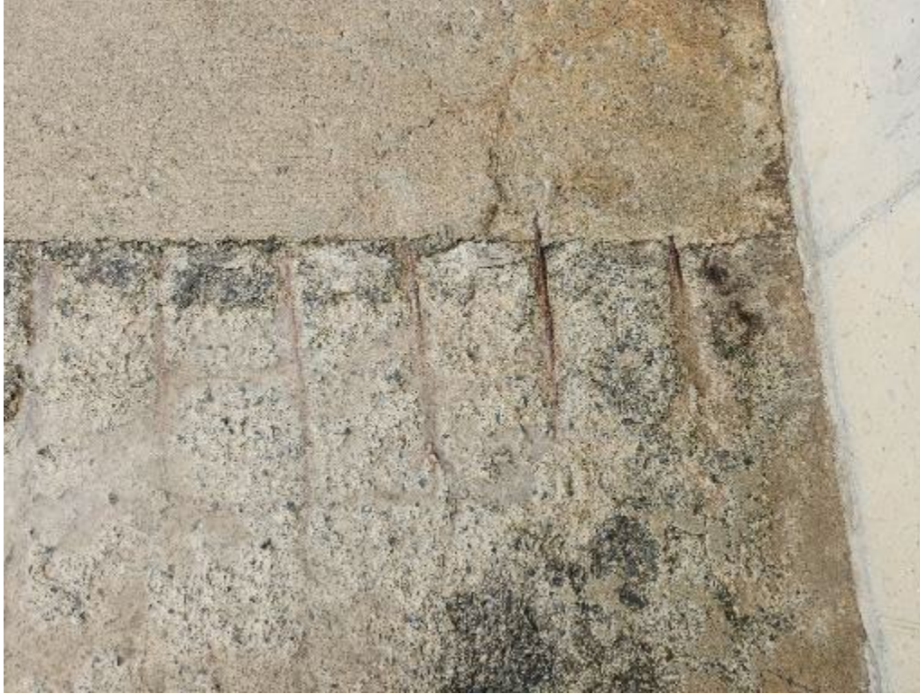
Photo 24: Rebar embedded at surface on south end of north dam crest
