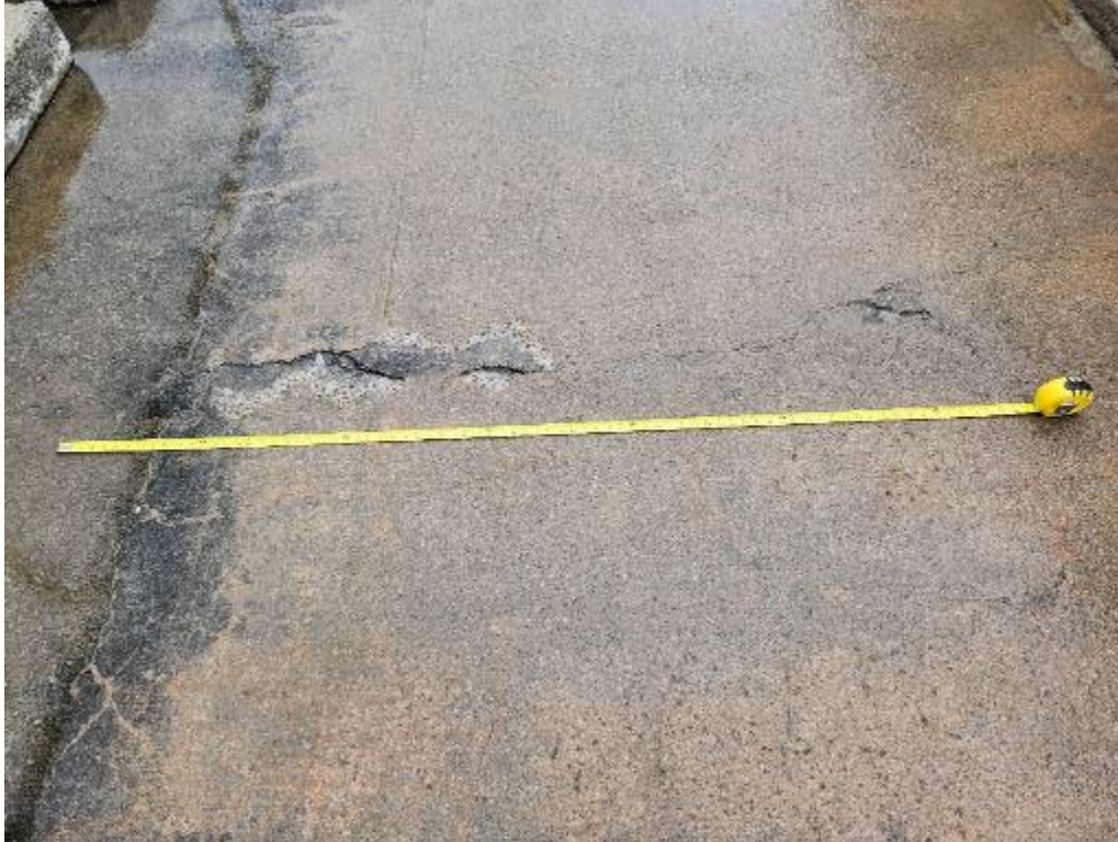
Photo 30: Delamination and cracking on dam crest
