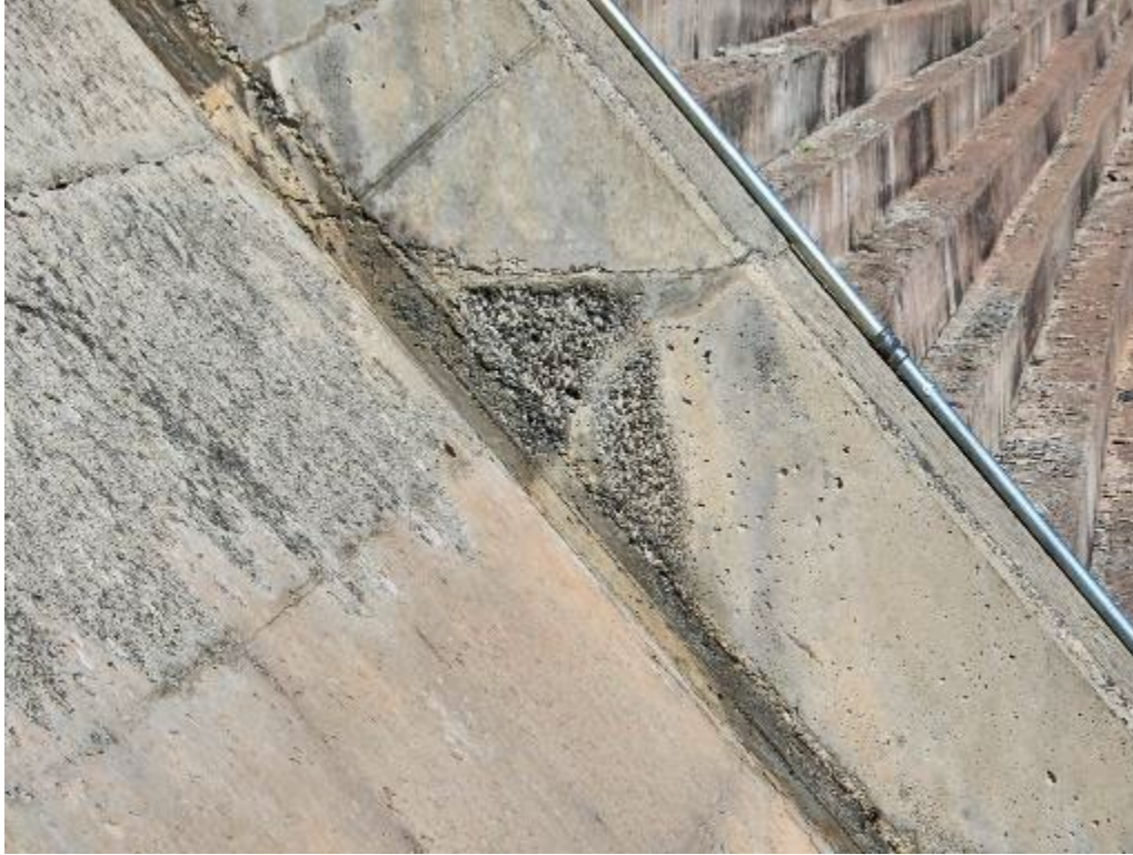
Photo 12: Poor consolidation and cracking on spillway left training wall
