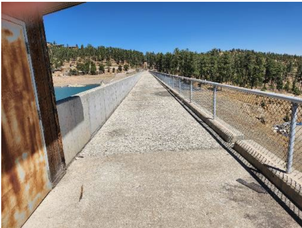
Photo 35: Transition from good to deteriorated concrete at south end of north dam crest
