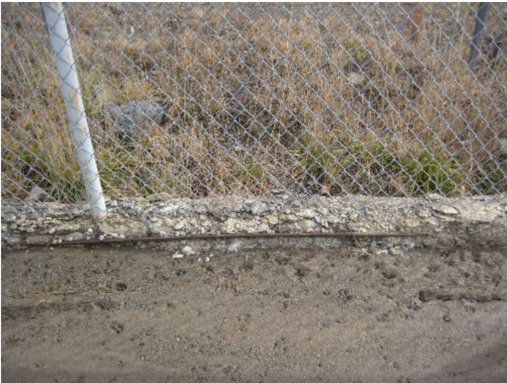
Photo 27: Deteriorated curb on north end of north dam crest
