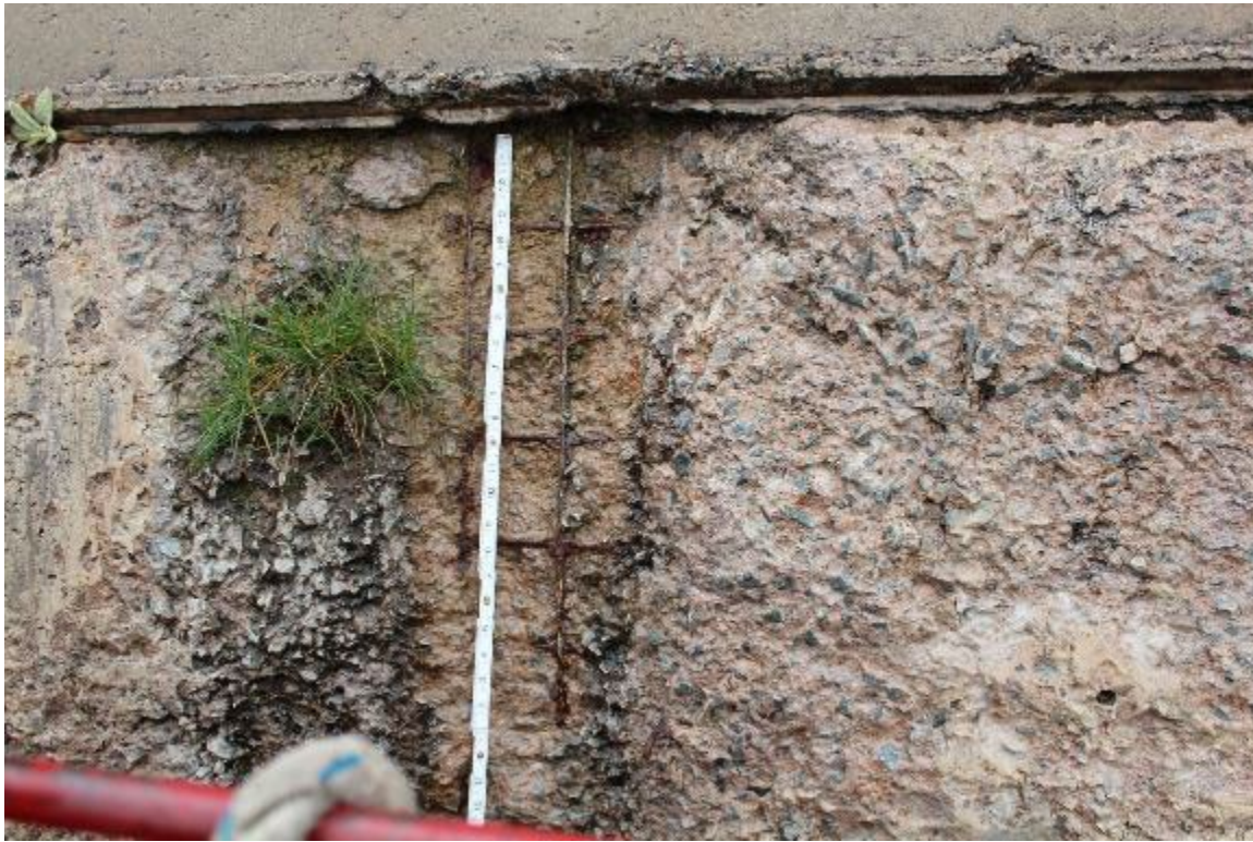
Photo 15: Exposed welded wire fabric at top of third facing element above bottom of spillway
