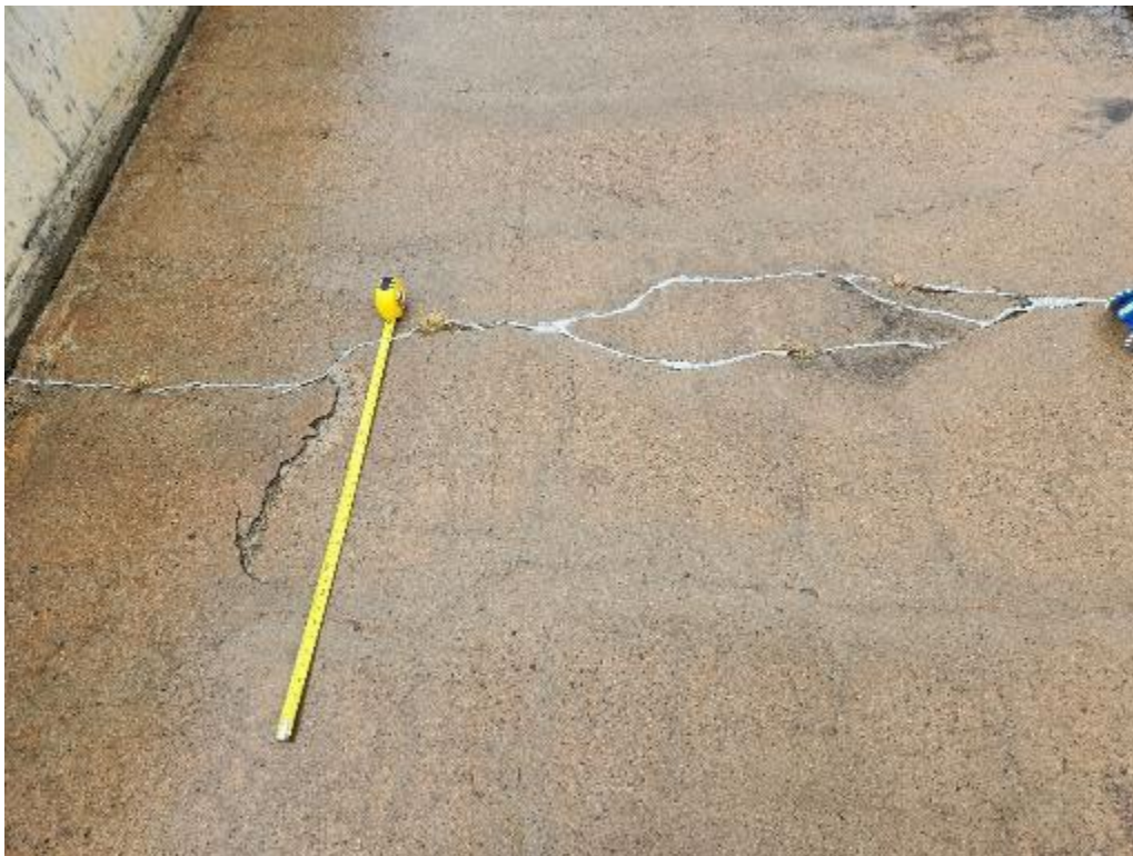
Photo 29: Delamination and cracking on dam crest, note previous caulking of crack with sealant
