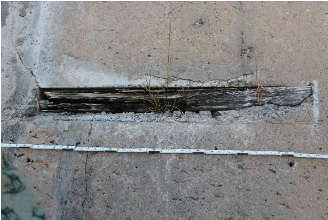
Photo 13: Wood embedded in concrete surface
