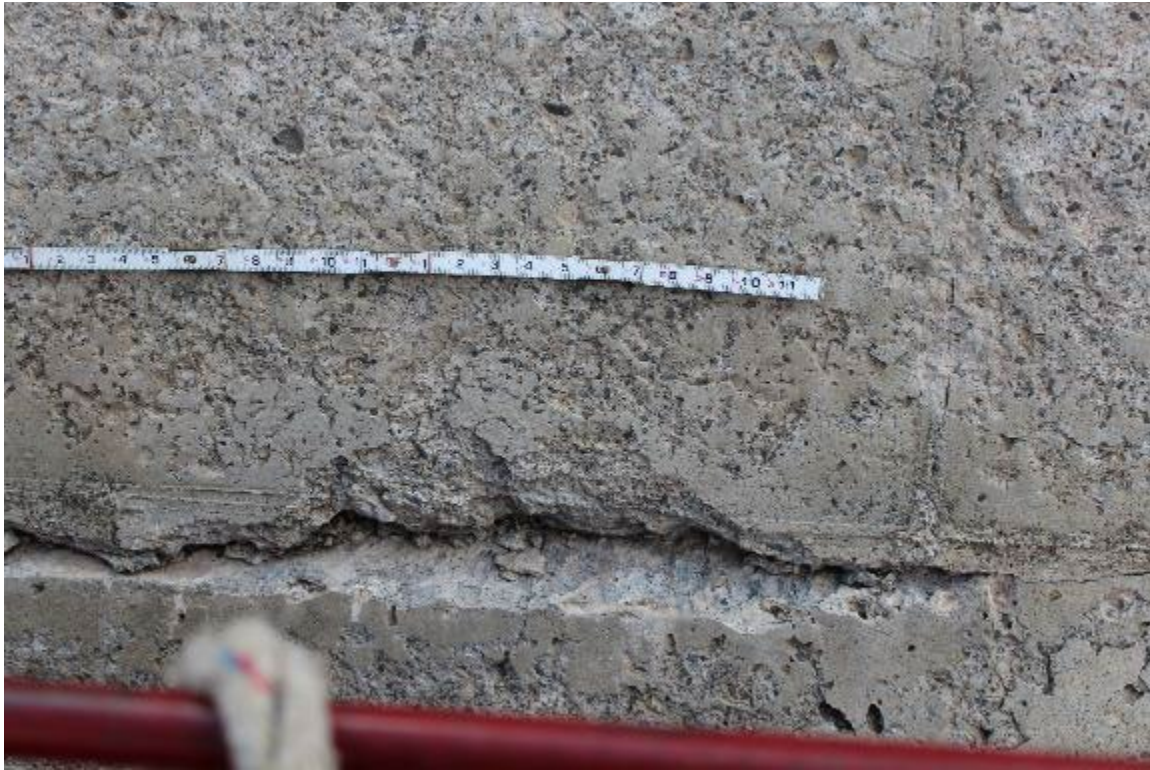
Photo 9: Spalling at horizontal joint on spillway
