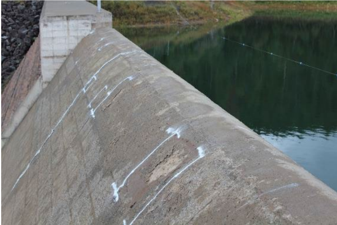
Photo 6: Delaminated areas on spillway crest
