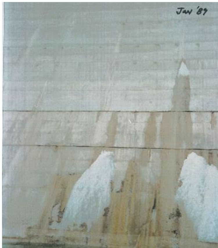
Photo 3: January 1989 Photo of Lower Right Spillway Surface
