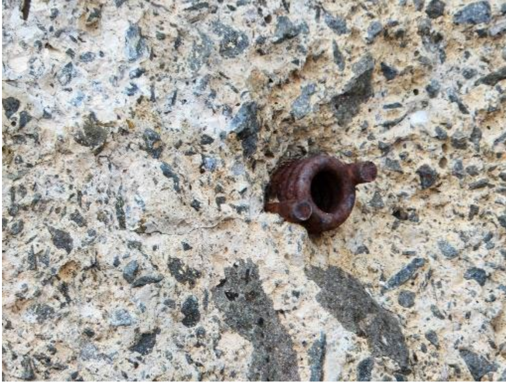
Photo 18: Exposed and rusted form support insert on spillway surface
