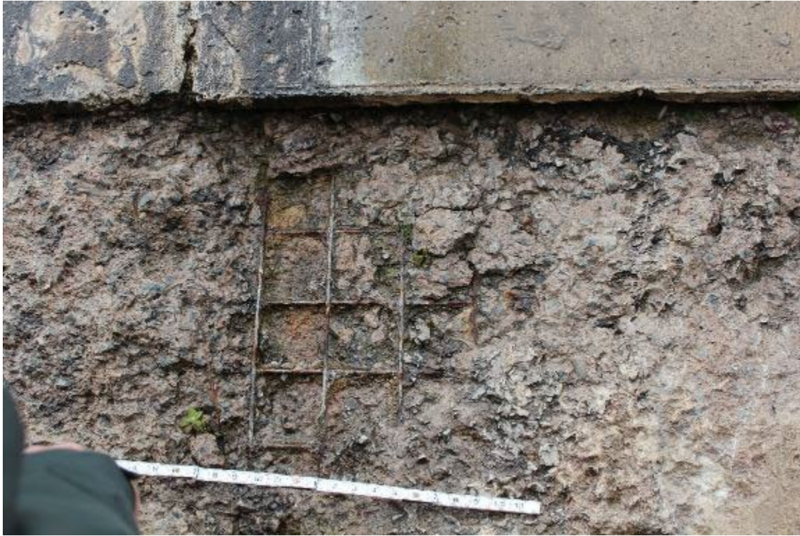
Photo 16: Exposed welded wire fabric at top of third facing element above bottom of spillway
